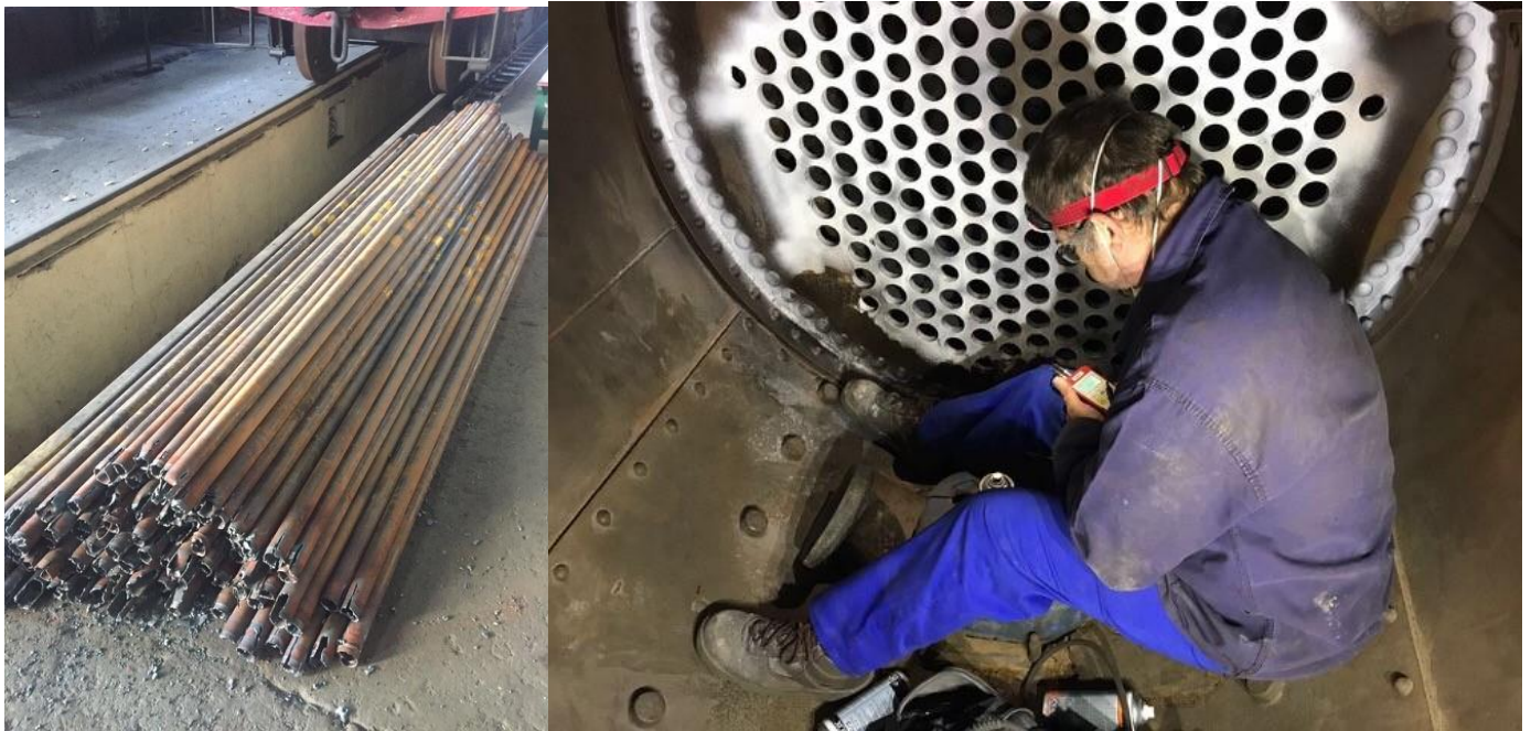
The tubes from 194 after removal and crack testing the boiler. Pictures from Reefsteamers.
